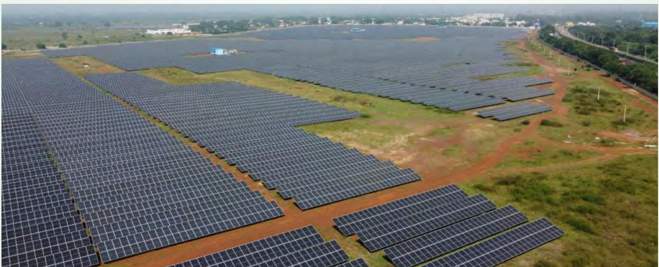
50 MW Solar power plant at Bhilai
