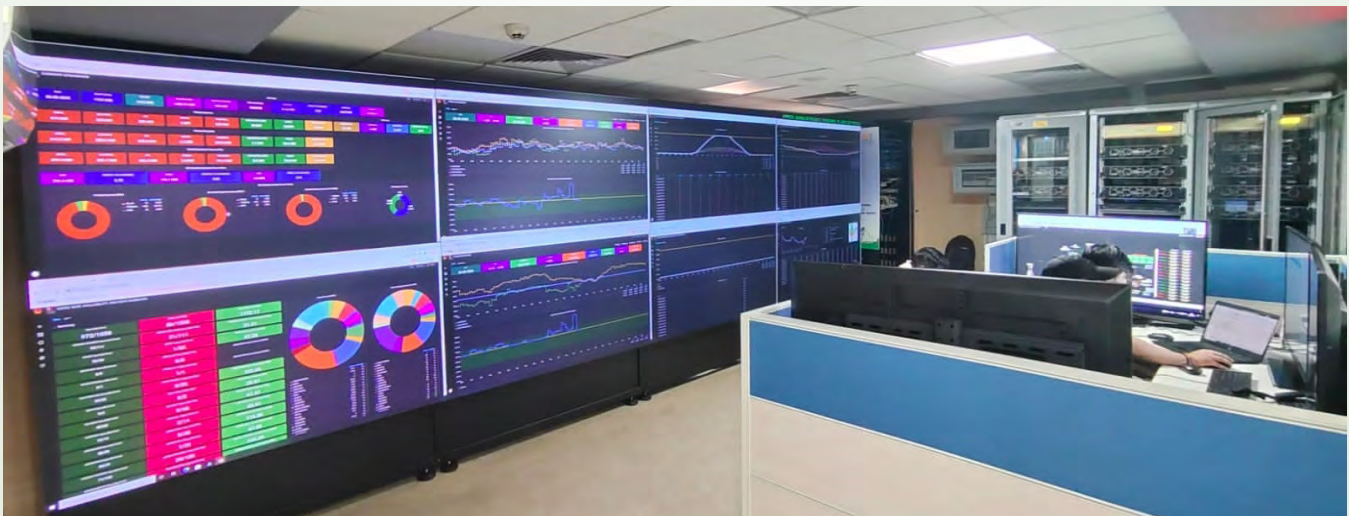
National Energy Management Centre (NEMC) at REMC, New Delhi
